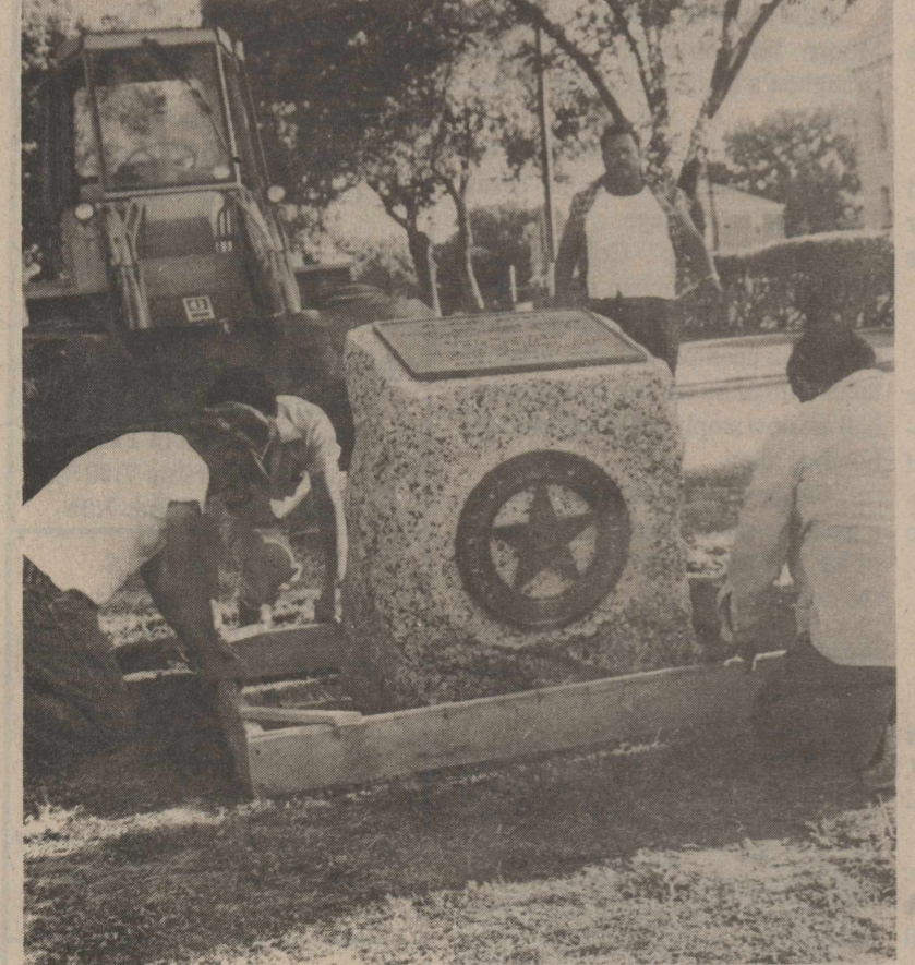
County workmen position a state marker commemorating Emerald townsite on the courthouse lawn Tuesday. Preliminary preparations for the marker placement, including a drawing, building forms for the base and digging the location, were done by Ricky Burger as a community service project in becoming an Eagle Scout. The marker has been in storage for a number of years after being removed from the roadside park east of Ozona when I-10 was built.
