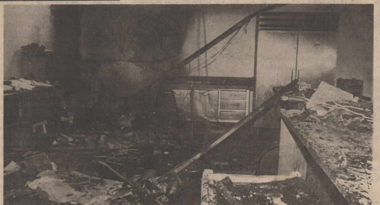
Chato Restaurant kitchen and upstairs office received extensive damage from an early morning fire Thursday. photo by Susan Sheppard
