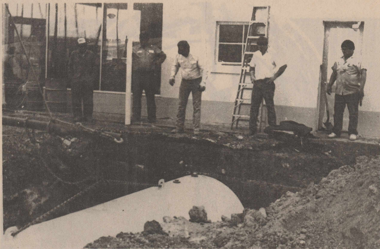
Chevron station operator Alfred Enriquez (right) watches as underground tanks are being removed to comply with EPA standards.
