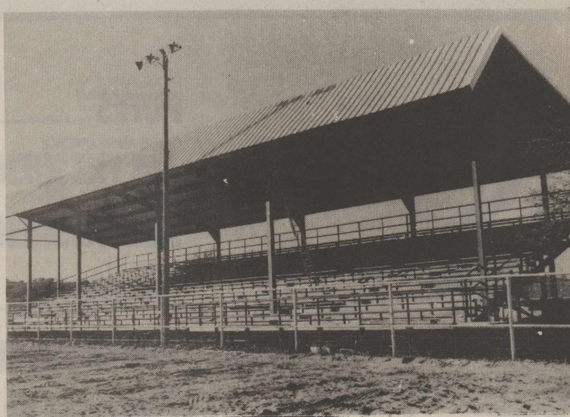
The grandstand at the rodeo arena has a new cover which was completed last week. The cover is a project of Crockett County Fair Association.
