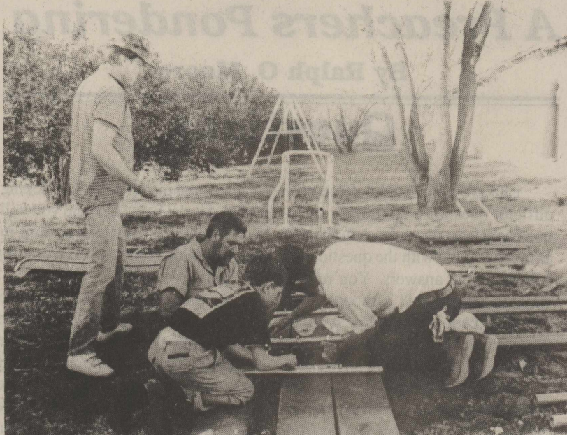
Pictured constructing playground equipment at Ozona Community Center last Thursday are: (l. to r.) Bill Fuller, Charles Preddy, Chris Gibson and Curtis Keith.
