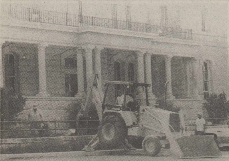
County employees were busy removing old shrubs from in front of the courthouse last week. The project is part of the centennial preparations.
