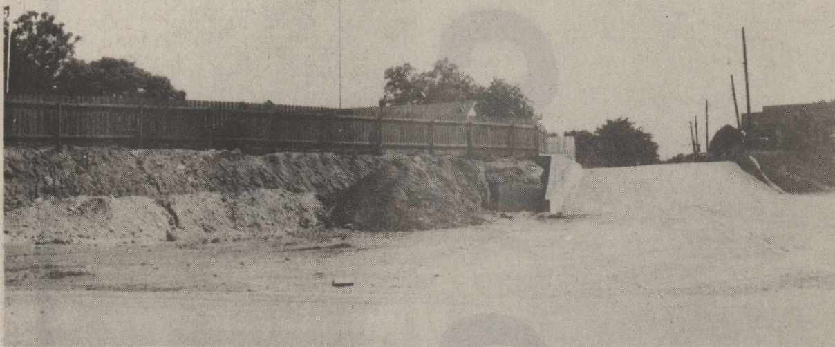
STREET AND CURB IMPROVEMENTS ARE UNDERWAY in Johnson Draw on Twelfth Street, adjacent to the Jim Caldwell residence. A new retaining wall has been erected and the junction of the two streets has been widened.
