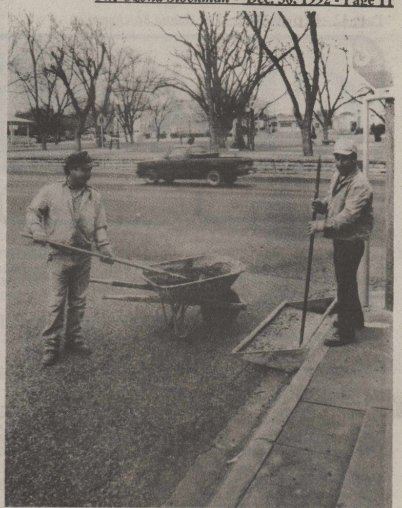
MALEO LUJAN AND ALBERT BORREGO, county employees, are hard at work installing handicap ramps in the downtown section of Ozona. Ozona Stockman photo
