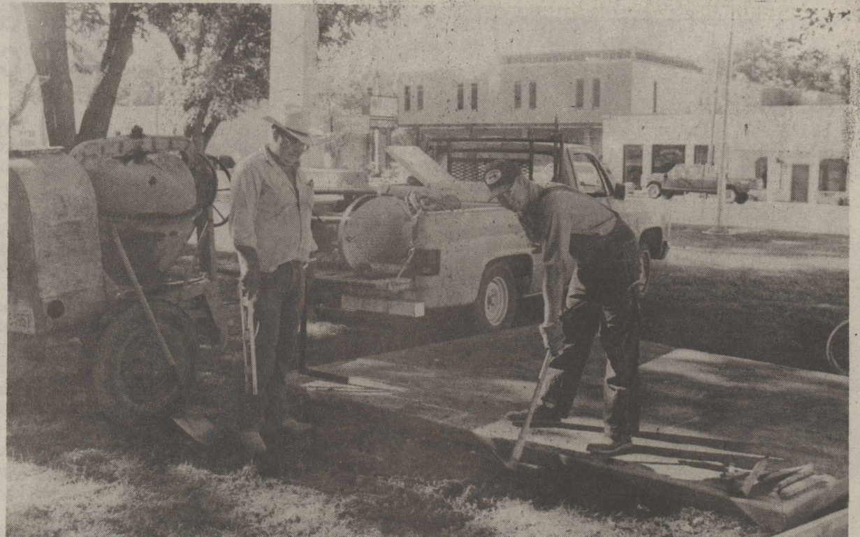
PREPARING THE BASE FOR THE LAST OF FOUR TRASH BARREL HOLDERS on the square Monday are county employees Sammy Hester and Richard Storms.
