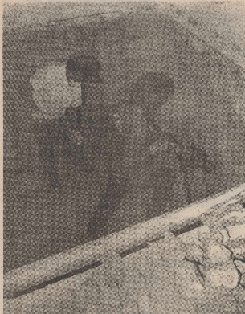
"RAT-A-TAT" goes the air drill as Travis Bond of Midland breaks off rock and James Adkins of Ozona shovels out rock and dirt. These men and others have spent two busy months in digging out five feet, four inches of rock in preparation for the elevator in the Crockett County Courthouse.
