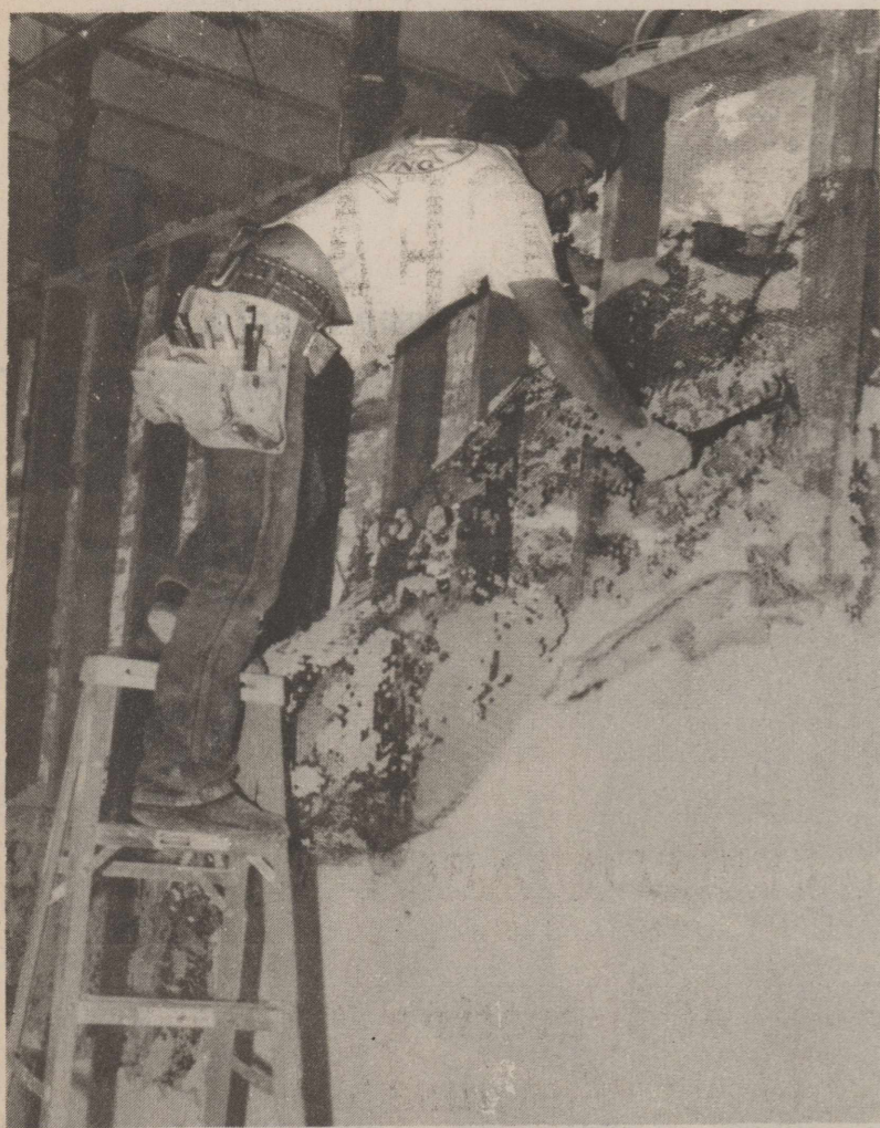
TONY NAVARRO of San Angelo works at ripping out a wall as part of the renovation at Crockett County Hospital. He is here with a crew from Mike and Vic Echert Building Contractors to prepare the building for conversion to a rural health clinic. Structural and electrical work began last week.
