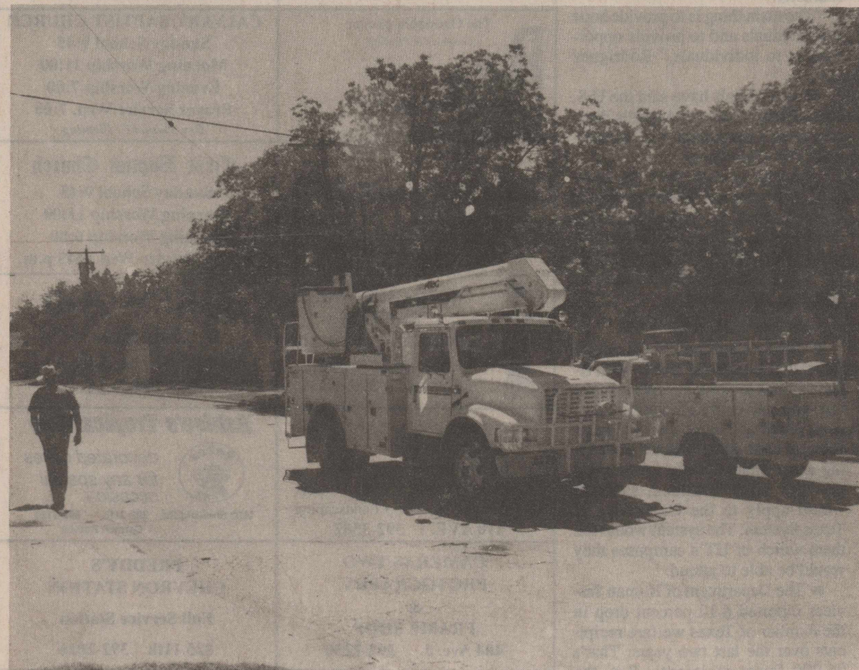
A WTU HIGH VOLTAGE LINE ON AVE. E burned into Sunday afternoon when it shorted out on a pecan limb. The hot wire fell to the ground and burned a large hole in the pavement just across from the post office before WTU workmen could shut off the juice. Ozona DPS officers and sheriff's deputies were kept busy stopping traffic while WTU linemen replaced it and restored power. photo by Scotty Moore
