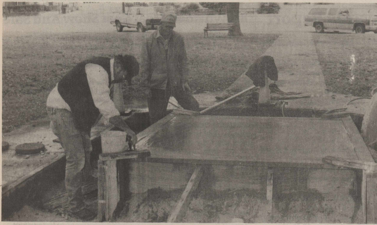
SMOOTHING OUT THE BASE for the Heritage statue to be placed on the square next month is Sam Hester. Richard Storms was also working on the project. photo by Linda Moore
