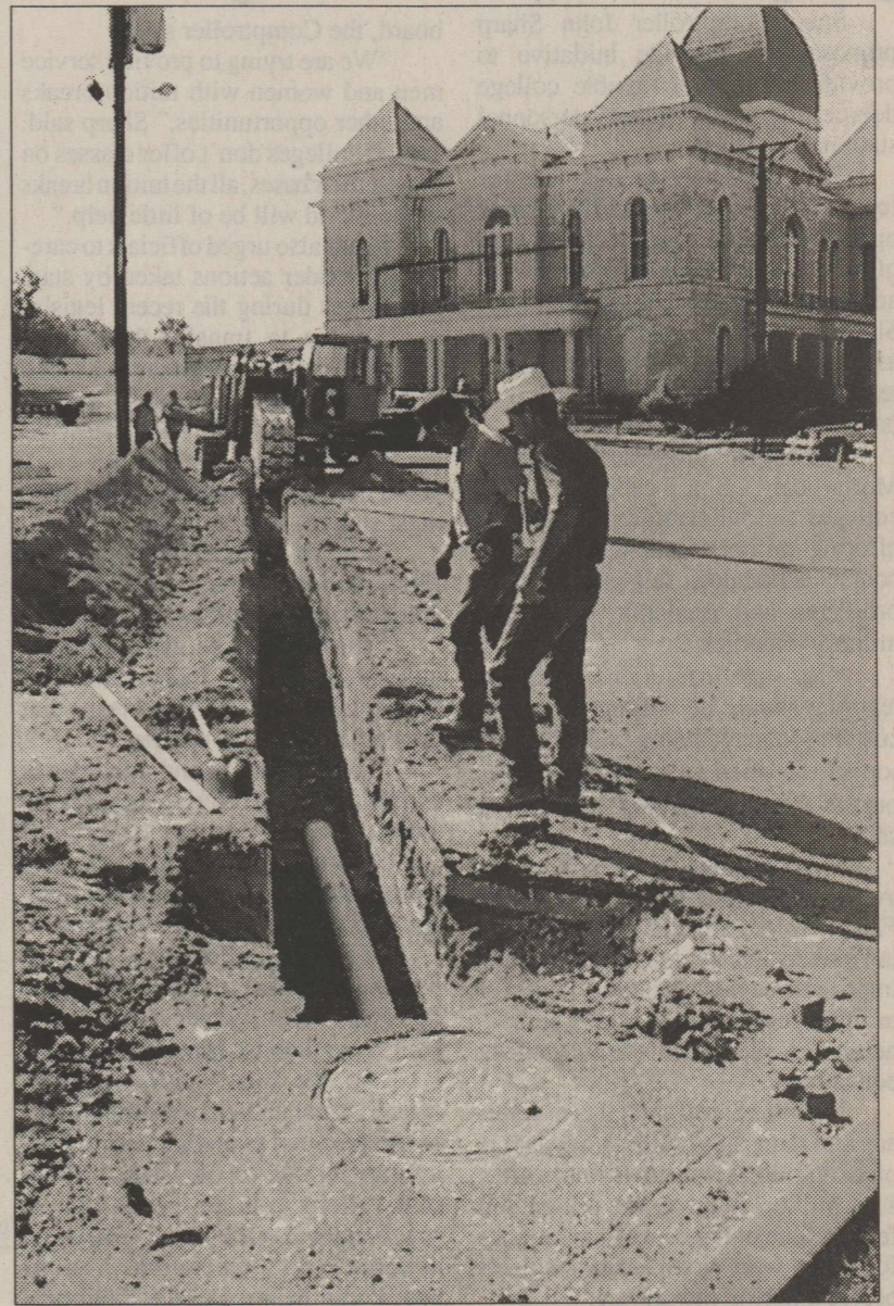
DOUG MEADOR AND DENNIS CLARK inspect the sewer lines which were laid Monday for the courthouse and the new annex building. DigiCam Photo By Scotty Moore
