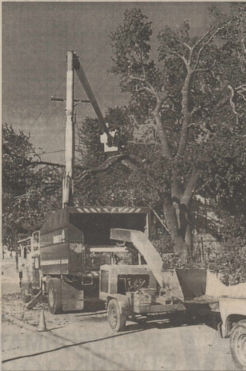
TREE TRIMMERS FOR WTU ARE BUSY AT WORK at the First Baptist parsonage. Radical trimming of trees around town has many residents up in arms. County Attorney Bill Mason says property owners can refuse to allow their trees to be trimmed. For information from WTU, see their ad on page 11. DigiCam Photo by Scotty Moore
