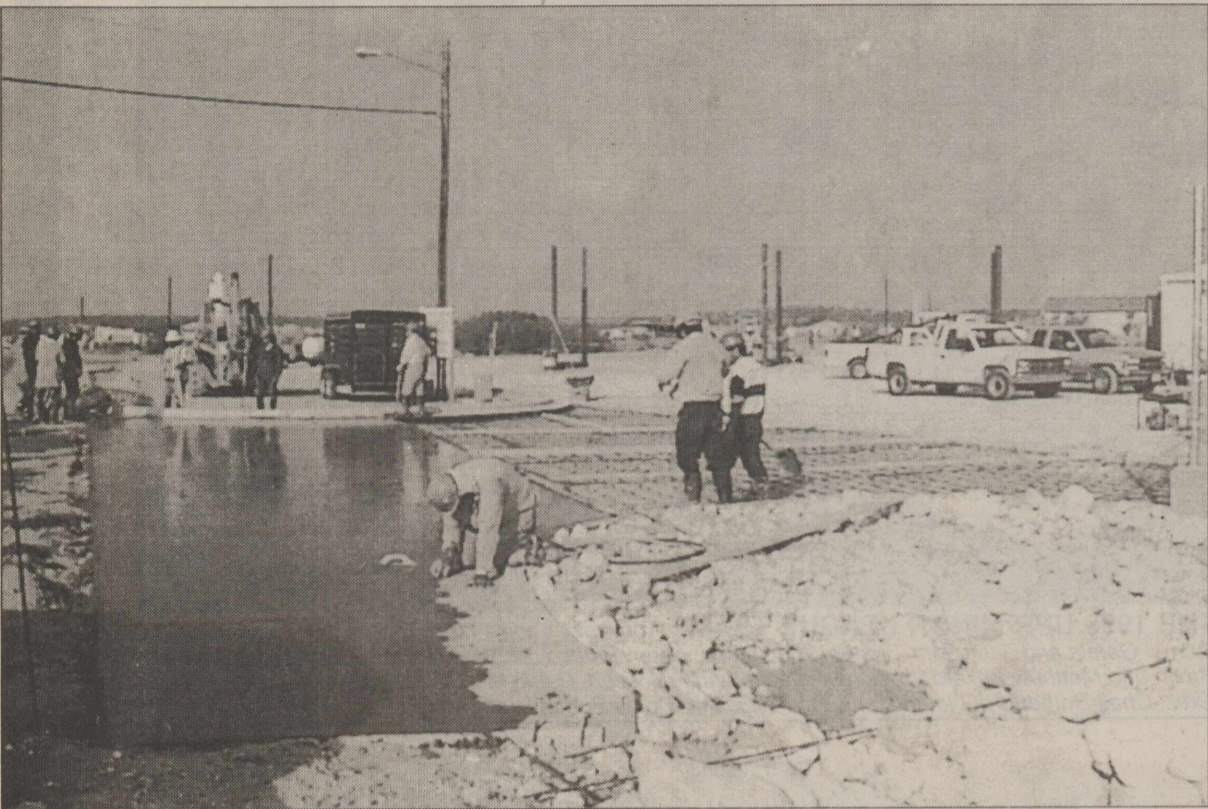
THE CONSTRUCTION AT THE NEW FRANK'S FUELS LOCATION on Hwy. 163 S. is shaping up nicely. Workers pictured here were busy smoothing cement last Wednesday. DigiCam Photo by Susan Calloway
