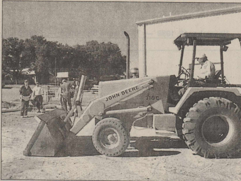
THE CROCKETT COUNTY YOUTH CENTER is eagerly awaiting the finish of the construction of the new concrete basketball area at the center. Pictured on the backhoe is county employee Estalfo Vargas. Richard Sanchez is the foreman of the project and he is assisted by this eager group of workers from the jail.
