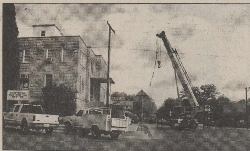
THIS CRANE BLOCKING ELEVENTH STREET last Wed., was removing the old air conditioning units in the museum building and placing new units for installation Photo by Scotty Moore
