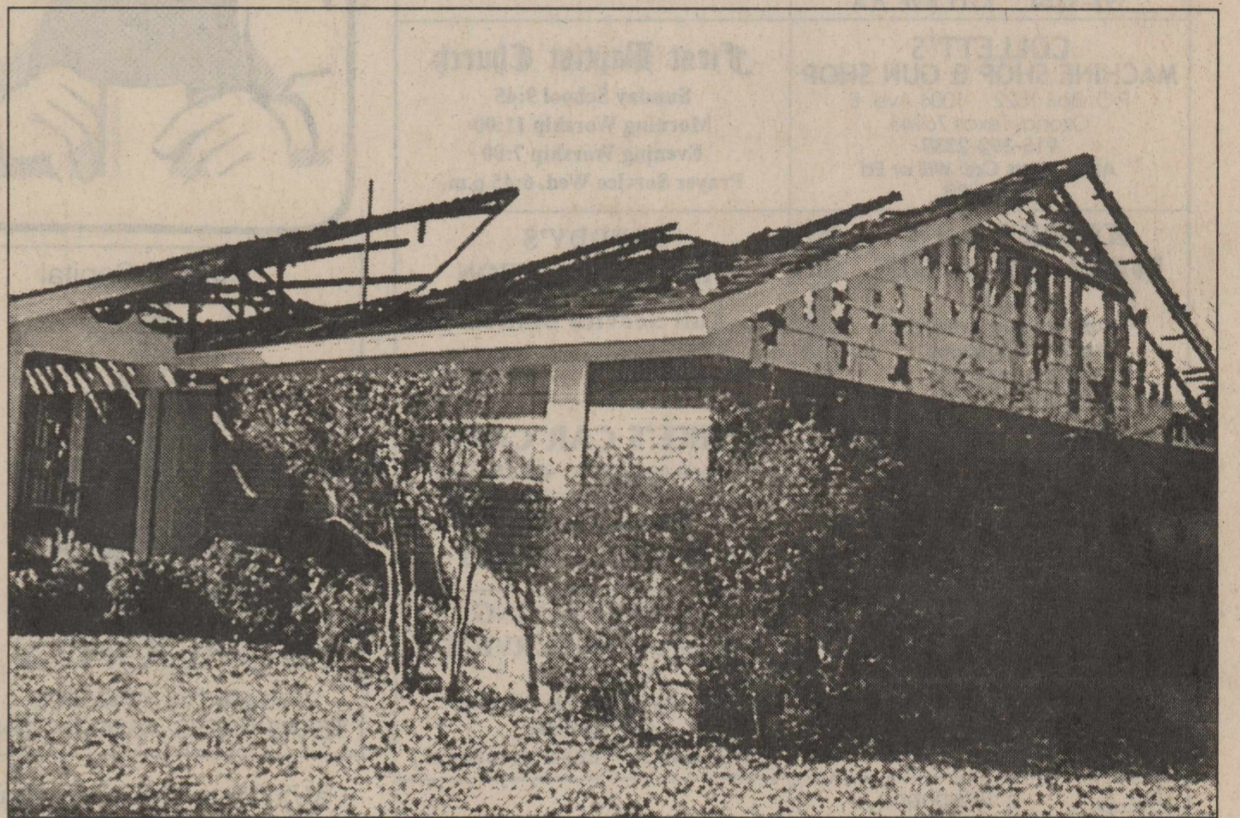
THE WOOD SHINGLE ROOF of Mrs. Jewel Bailey's home at 1001 Henderson Drive was destroyed by fire in the early hours of Jan. 1. Photo by Scotty Moore
