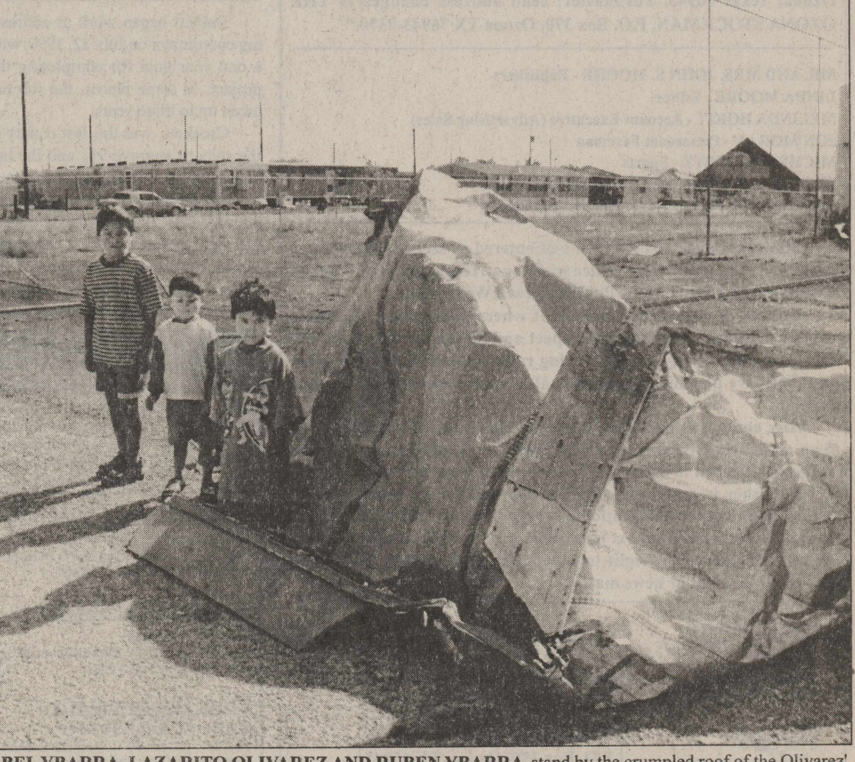
ABEL YBARRA, LAZARITO OLIVAREZ AND RUBEN YBARRA stand by the crumpled roof of the Olivarez' mobile home which blew off in a storm May 27.
