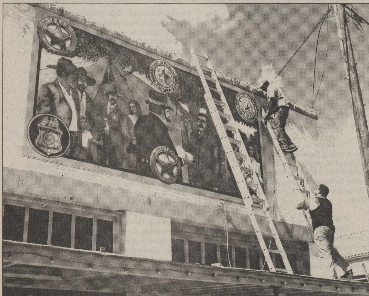
SECURING THE NEWEST MURAL on the Perry Building are Refugio Chipman and Jacob Lara of Lara Construction. Commissioned by Gene Perry and painted by Alfredo Tobar, the mural is a tribute to the branches of law enforcement which have served Crockett County. photo by Scotty Moore
