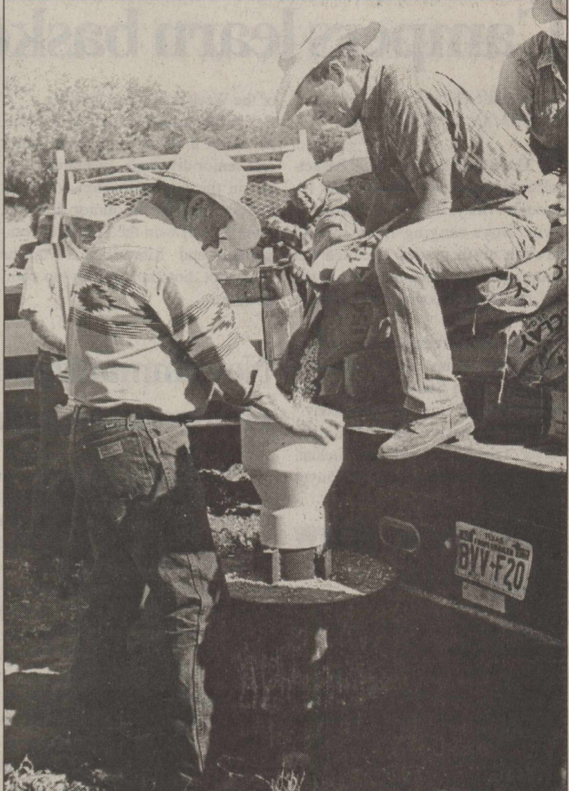
DENNIS CLARK , (r.) Emerald UWCD manager, pours specially prepared clay into an abandoned water well. He is assisted by Virgil Poloccek, assistant manager for the Sutton County UWCD. Observing in the background of the TAMU Extension Service and Underground Water District's abandoned well plugging demonstration are: Troy Williams (l.) and Nat Reed. Photo by Stephen Zuberbueller
