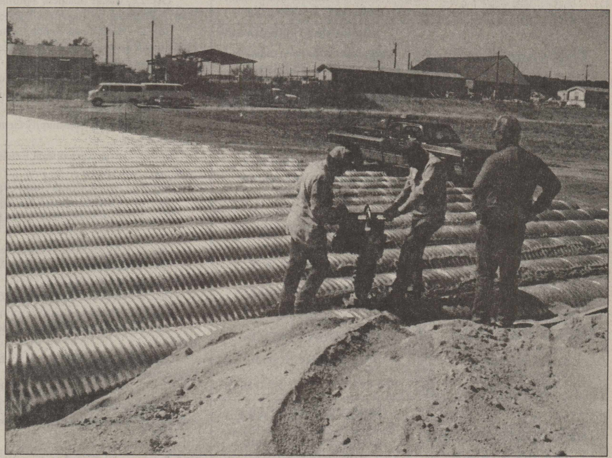
EDDIE MOORE, road superintendent (r.) checks on construction of the bridge across Johnson Draw at War Admiral Street. Tamping sand between culverts are Adam De La Garza and Willie Payne. DigiCam Photo by Linda Moore
