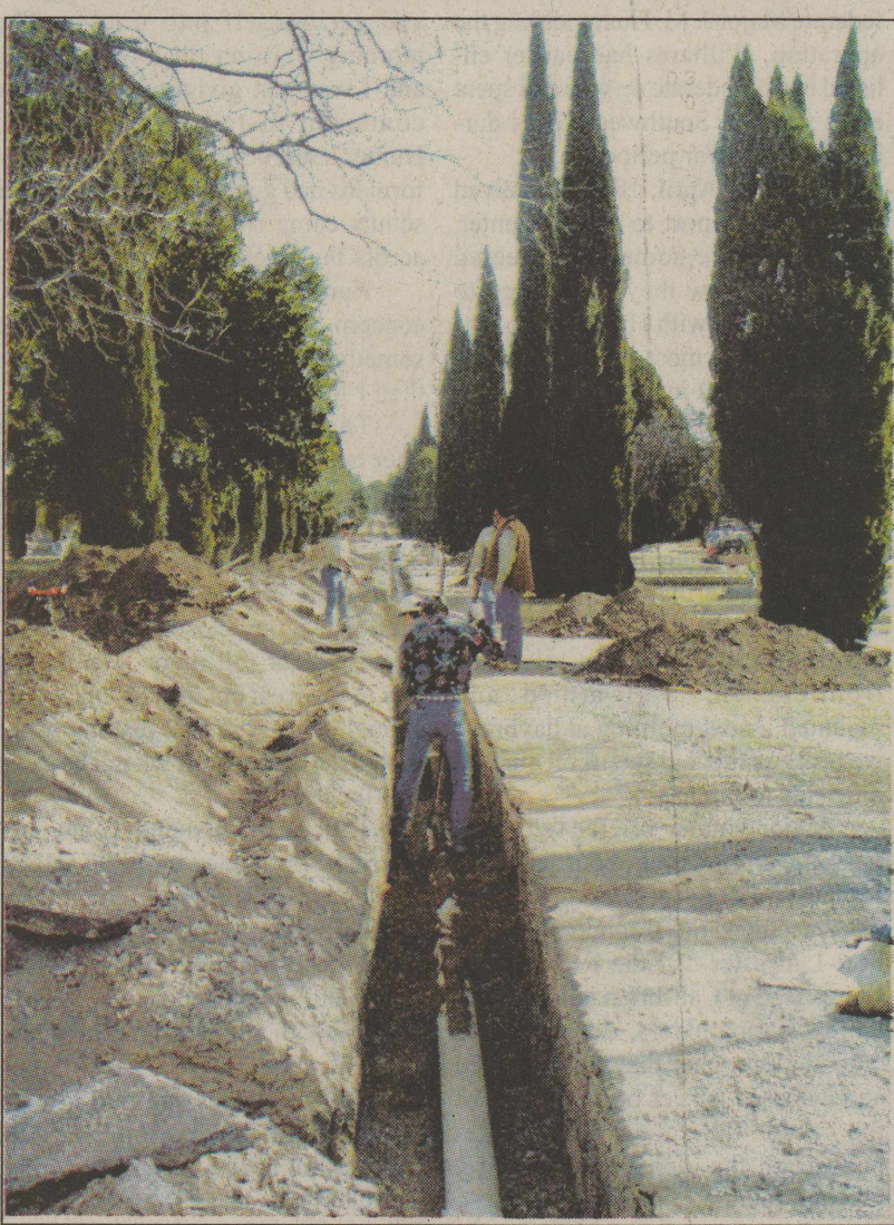
A SIX-INCH WATER LINE IS NOW IN PLACE from one end of Cedar Hill Cemetery to the other. Estimated to take two months to complete, the new watering system will work on timers. Excavation for placement of lateral lines began this week. DigiCam Photo by Scotty Moore
