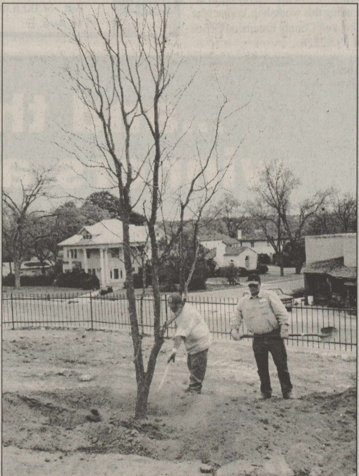
CROCKETT COUNTY ROAD DEPARTMENT employees Tooter O'Bryant and Israel Guevara shovel in dirt onto the red oak tree being planted on the south side of the annex building. Also being planted are two live oaks, three fruitless pear trees and 36 ligustrums.
