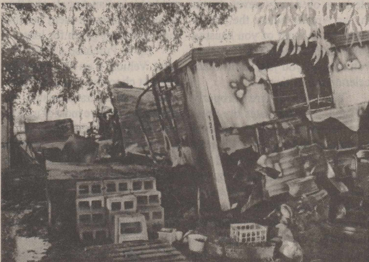
Submitted photo and photo by Joe Hernandez TOP: OZONA VOLUNTEER FIRE FIGHTER GIL KOMECHAK fights the fire between the two mobilehomes Monday on Willow Street. BELOW: The remains of the mobile home after the firefighters cleared the scene.
