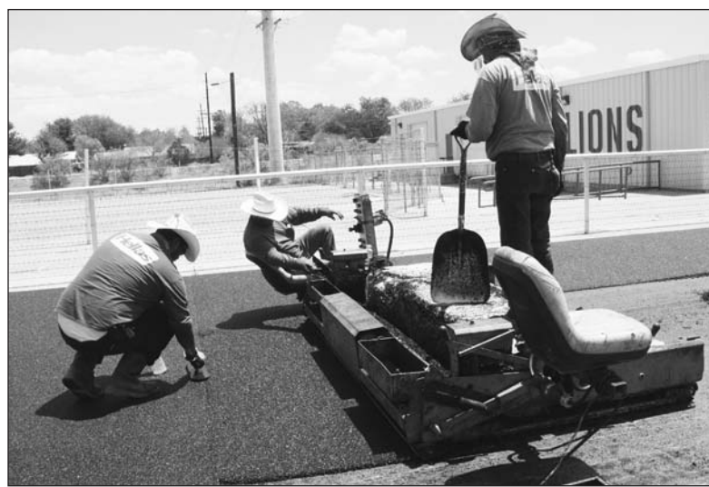
JOE HERNANDEZ | THE OZONA STOCKMAN EMPLOYEES OF HELLAS CONSTRUCTION layout the foundation Monday of the new track at Lion Stadium. The work being done at Lion Stadium is being paid for through the Qualified School Construction Bond program.
