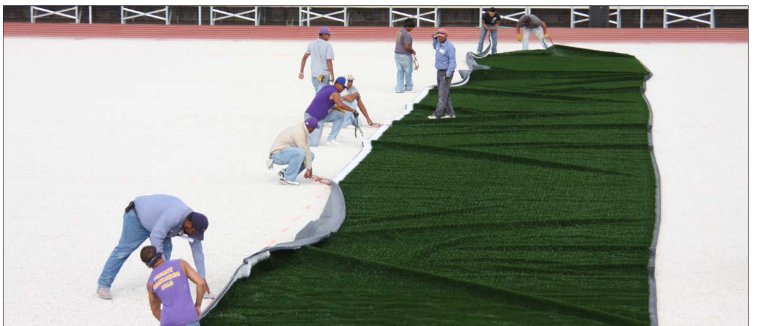
WORKERS STARTED LAYING OUT the rolls of bright green artificial turf last week at Lion Stadium. Carter Construction is overseeing the project which is running on schedule to be completed by the time football season begins next month.
