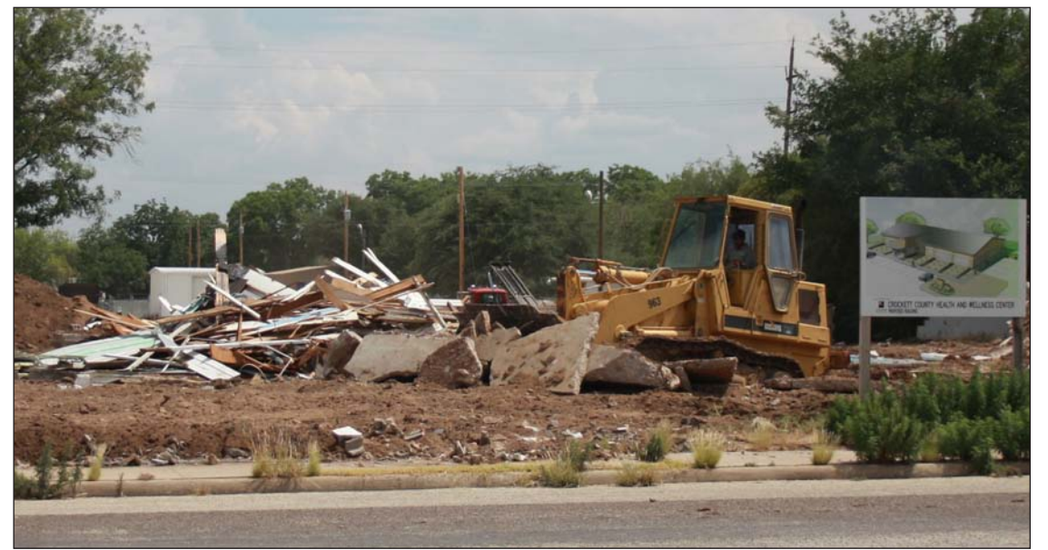
CROCKETT COUNTY EMPLOYEES TEAR DOWN the remains of the North Pool last week. The pool, located across from Lion Stadium, is the site of the future Crockett County Wellness Center. Until the center is built, the county and wellness center board members have agreed to allow CCCSD to use the site as a parking lot.
