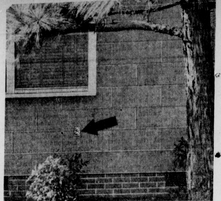
A weatherproof receptacle (arrow) near the front entrance makes it easy to use your electric lawnmower in addition to providing a safe means of lighting your Christmas decorations.
