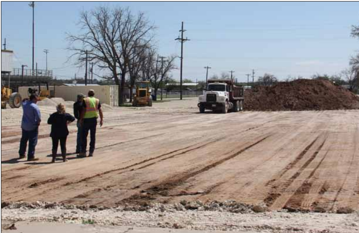
WORK ON THE NEW HEALTH CLINIC began Monday. The $3 million facility will be located across the street from Lion Stadium. It will include new equipment furnished by Shannon Medical Center. Frontera Construction, of Del Rio, is building the clinic. The building is estimated to be completed by November.
