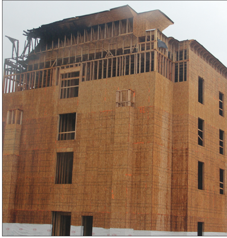
JOE HERNANDEZ | THE OZONA STOCKMAN THE NEW HAMPTON INN that is being constructed on 14th Street caught fire after lightning struck the building Sunday night.
