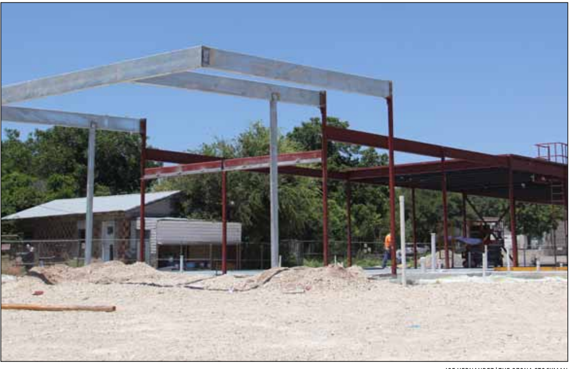
CONSTRUCTION ON THE NEW OZONA CLINIC continues. The clinic is located across from Lion Stadium. During a special meeting Monday, the Crockett County Commissioners' Court approved the first interest payment on the clinic's tax notes.
