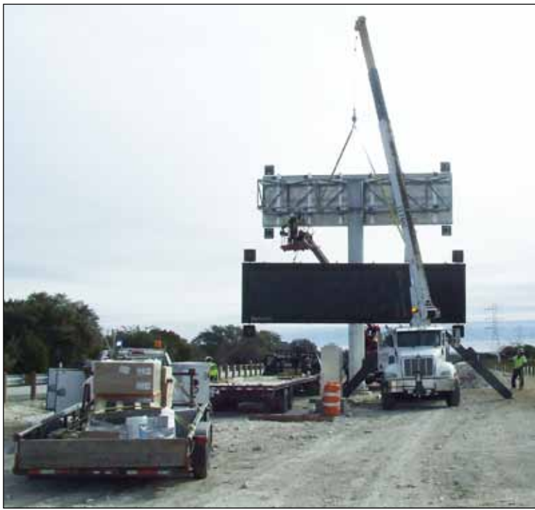
INSTALLATION OF OVERHEAD PERMANENT MESSAGE SIGNS is taking place along Interstate-10 by the Texas Department of Transportation.
