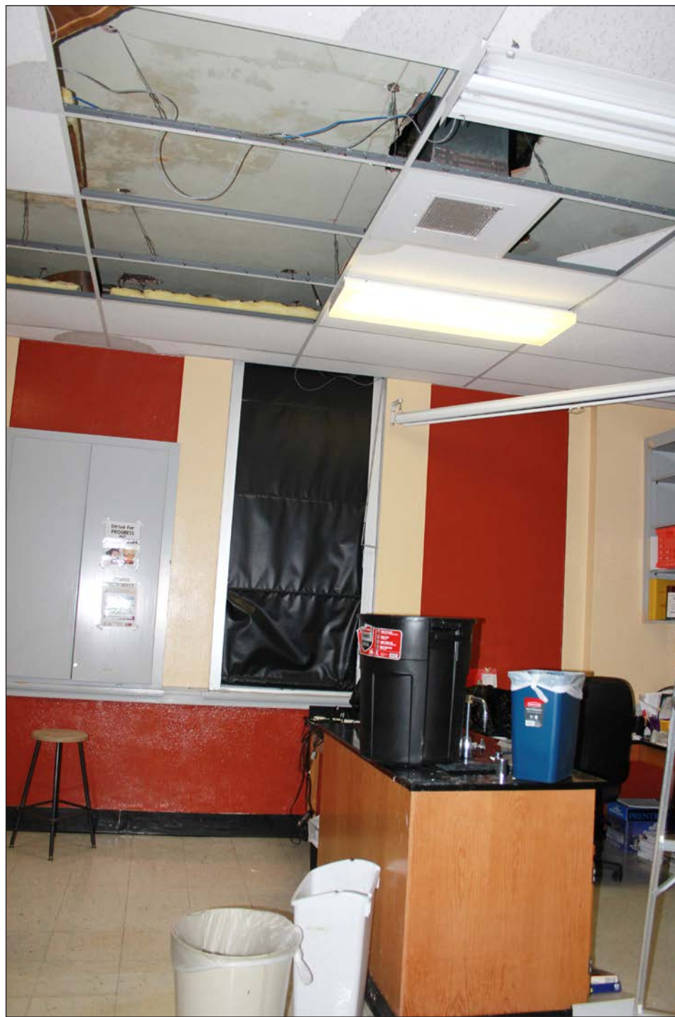
TRASH CANS and buckets collect water due to roof leaks in a third floor science lab of the OHS Main Building. Roof leaks have caused classes to be moved to other buildings.
