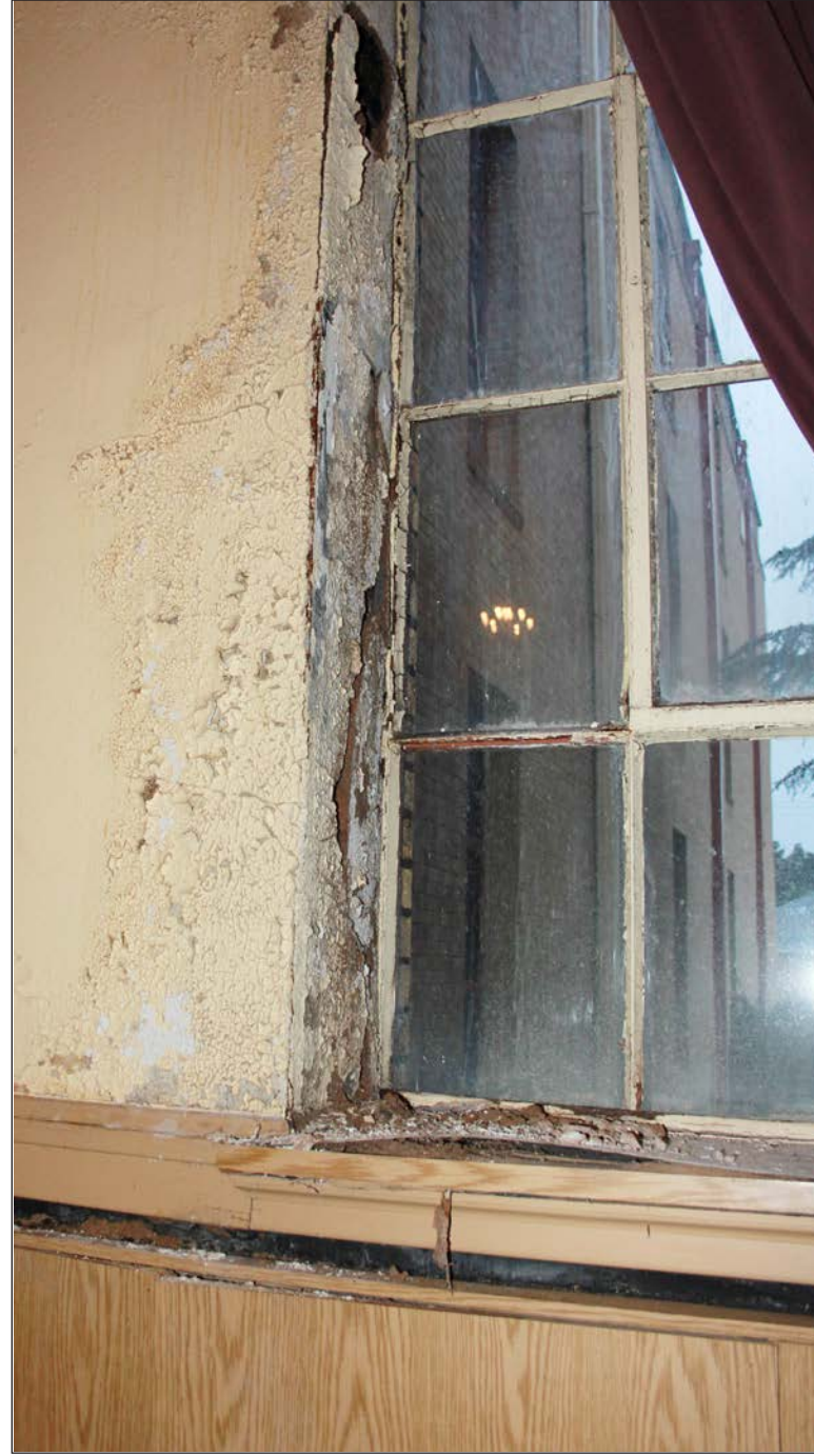
ONE OF THE WINDOWS in the OHS Auditorium that has sustained severe water damage. The OHS Auditorium is currently closed.
