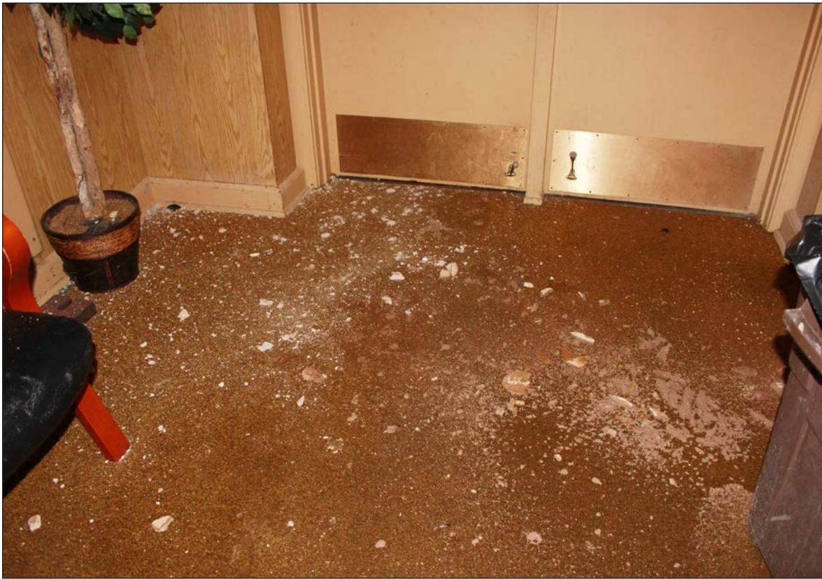
PARTS OF THE OHS AUDITORIUM CEILING has fallen onto the floor outside one of the doors.
