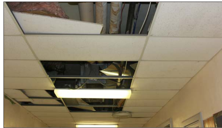
CEILING TILES in a hallway of the OHS Main Building have been stripped away due to water damage revealing insulation, wiring and conduit.
