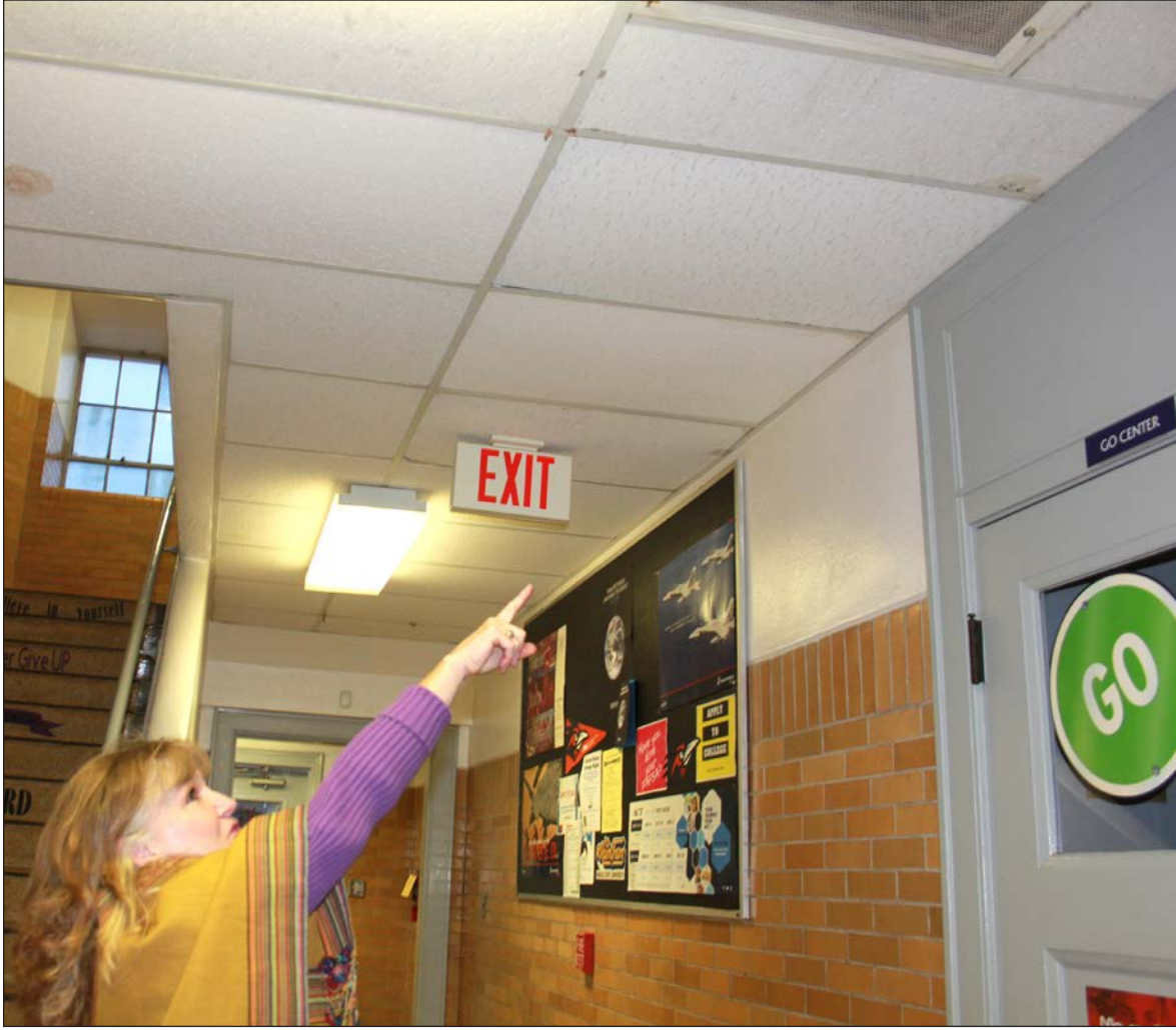
OZONA HIGH SCHOOL PRINCIPAL TAMMY MCWILLIAMS points to a leak in a new ceiling tile outside the OHS Office in the Main Building on Oct. 18.
