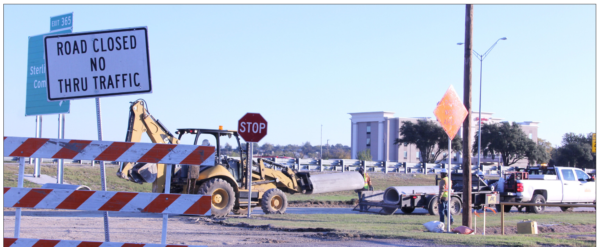
EMPLOYEES WITH ALLEN KELLER COMPANY start the concrete work on the Interstate-10 Frontage Road Extension Project Tuesday morning. Due to construction, part of the Frontage Road that runs by the 365 exit in front of El Chato's Restaurant down to Stripes Convenience Store and the Swimming Pool Park will be closed to traffic. The 365 exit was still open for off coming traffic. The road will be converted into a one way during the project. Work on the project began Oct. 15 but was delayed 16 days due to weather. The $3.4 million project is expected to take about a year to complete. The project is being overseen by the Texas Department of Transportation.
