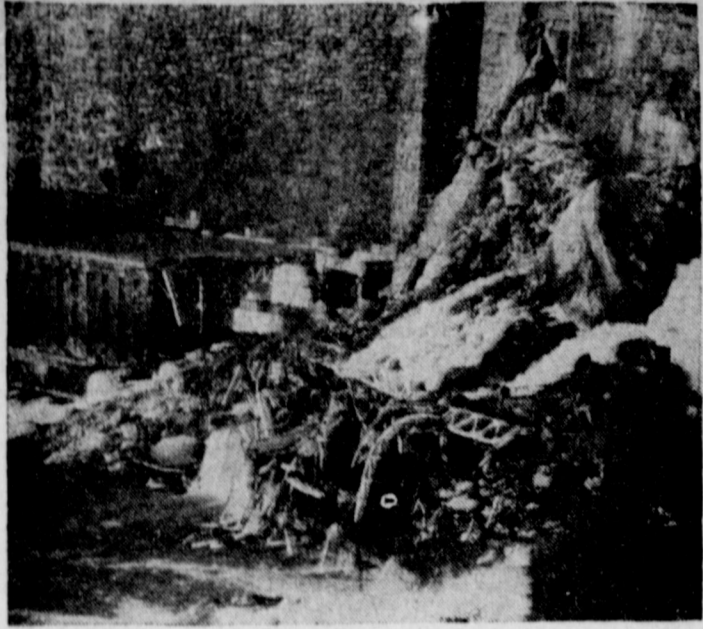
POWER STATION SLIDES INTO NIAGARA — Three earth-jarring slides left most of the giant Scholckopf power station in Niagara Falls, N. Y., in complete ruins. It was the largest Hydroelectric power facility in the Niagara Mohawk system. One man is dead and the damage will run into the millions. The industrial city of Niagara Falls, with its population of 100,000, was without electrical power for two hours. The spectacular collapse was caused apparently by seepage of water and "earth movements" in the area.
