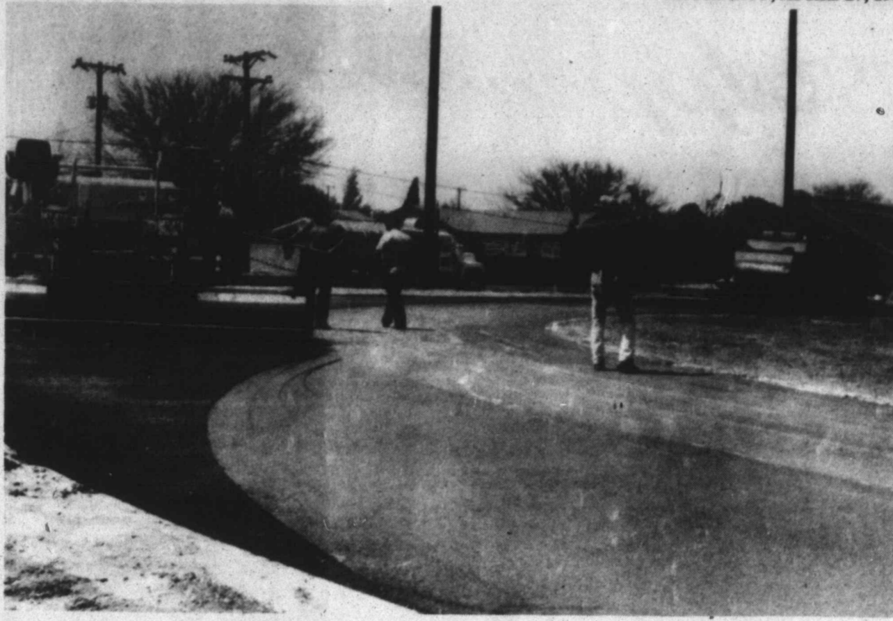
BRING IT THIS WAY - Work continued on the Tahoka High School track this week, with the track due to be completed sometime in May. Armor Asphalt of Lubbock is doing the construction of the seven-lane track. (LCN PHOTO)
