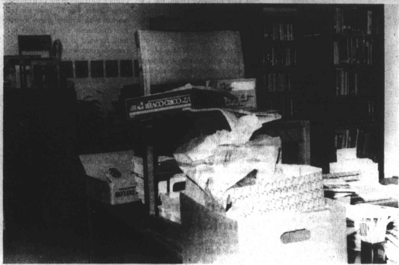
MESS AT THE LIBRARY —A faulty water heater burst early Sunday morning at the Life Enrichment Center, spewing water over walls, carpet, books and other materials at the City-County Library. This view shows the circulation desk and other areas stacked with furnishings as industrial air blowers were used to dry the carpet. The storage closet at the library was directly underneath the water heater, and walls and ceiling tiles also sustained some damage. The library will remain closed this week until repairs can be made, but librarian Shirley Draper noted that books may be returned at the outside book drop. It is hoped that repairs will be made and the library restored as soon as possible, possibly next week, but patrons are asked to call first to make sure the library is open before planning a visit. (LCN PHOTO)
