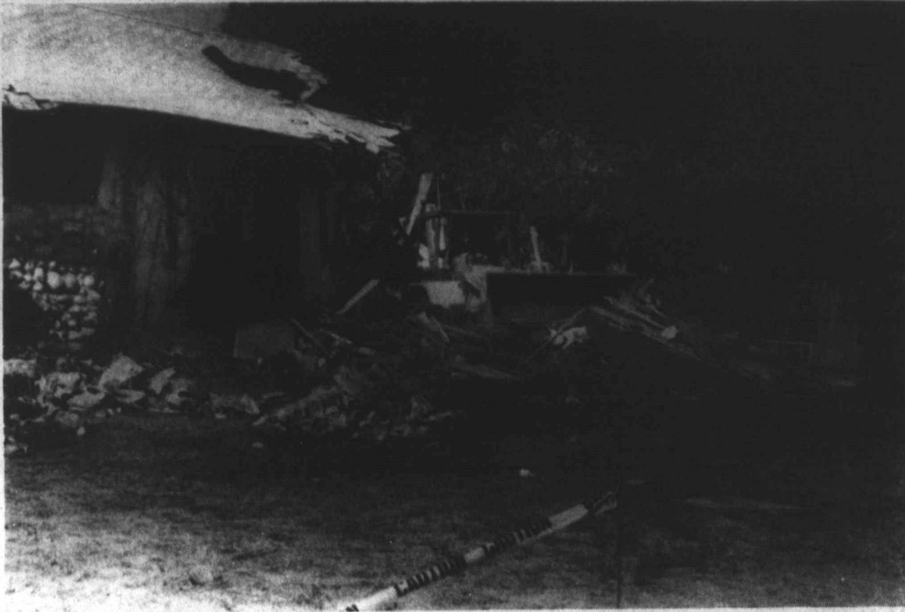
DEMOLITION PROJECT - City of Tahoka workers demolish the old Community Center on South 1st Street this week, tearing down the condemned building. This photo was taken early Monday afternoon, as workers bulldozed the north side of the building. (LCN PHOTO)
