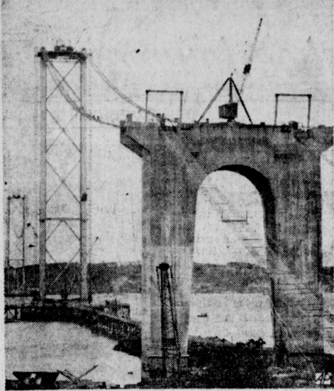
FORTH SPAN —Cables are strung from the twin steel girder towers of new suspension bridge rising across the Firth of Forth at South Queensferry, Scotland.
