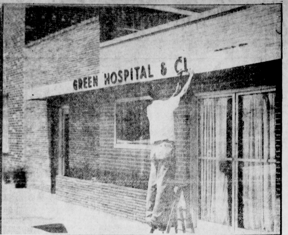
A NEW FACE FOR THE HOSPITAL — a workman is shown above as he places lettering on the front of Green Hospital and Clinic. He also installed a nameplate beside one door and a caduceus, the medical insignia made up of the winged staff of Mercury entwined with serpents, beside the other.
