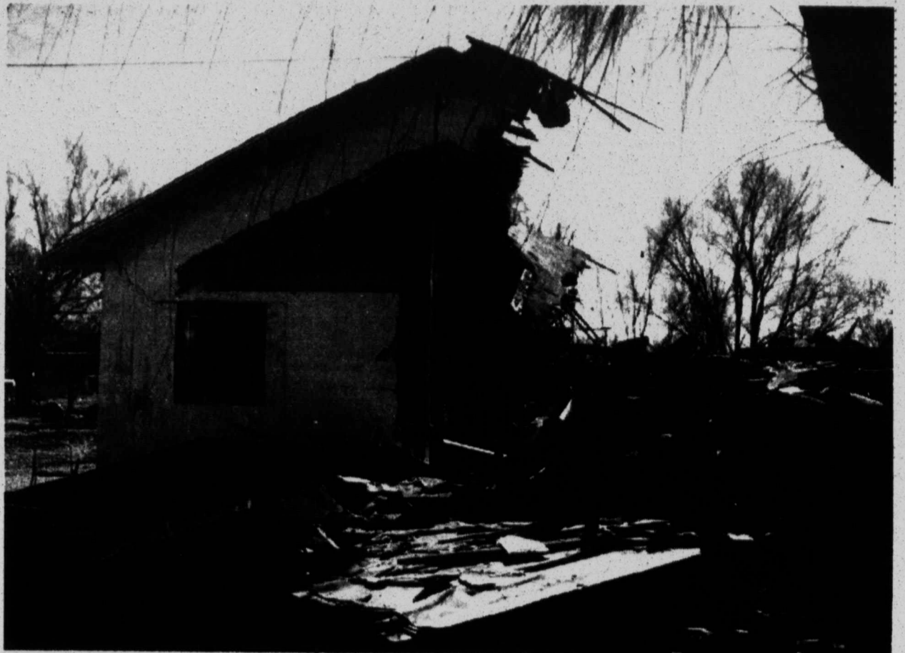
AND THE HOUSE CAME TUMBLING DOWN — City of Tahoka workers recently demolished the home of Esther Green, at 1115 N. 5th, in preparation for her new ready-built home to be moved in. Mrs. Green is one of three homeowners getting a new 2-bedroom home at no cost, through the City of Tahoka's HOME grant program. (LCN PHOTO)
