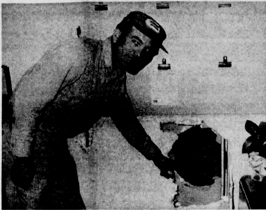
KENNETH GEORGE of Baker Farm Supply Monday night, with property damage the points to hole made by burglars between the Baker store and Patzer Clinic. Burglars forced their way into four Muleshoe stores
