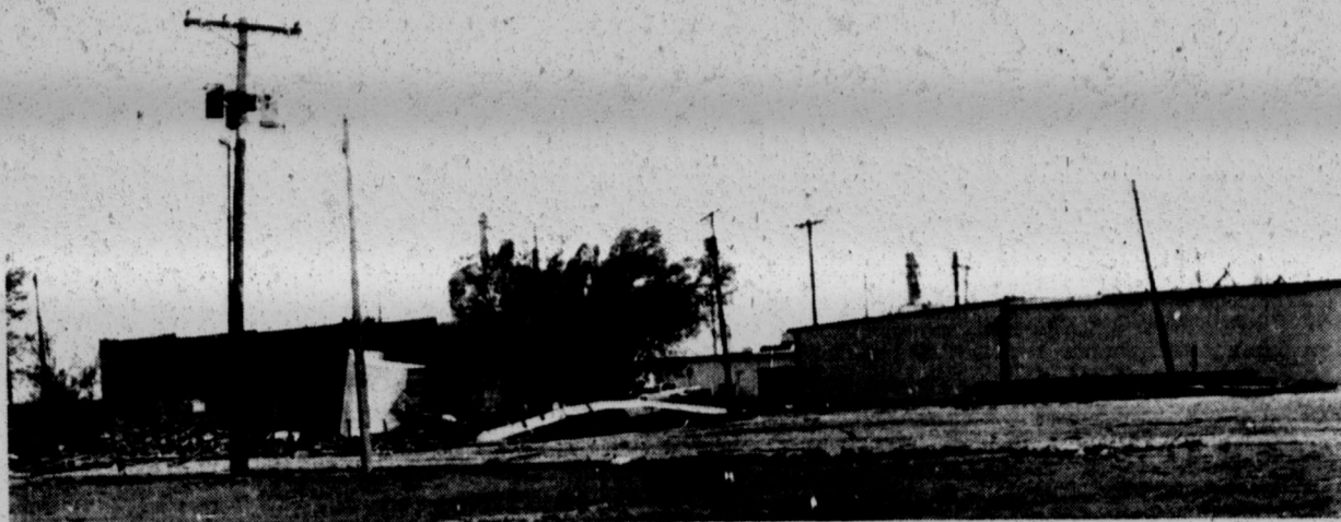
STORM DAMAGE - This building behind the Green Mercantile building at Wilson sustained damage during a March 25th afternoon storm in the county. The roof of the building was lifted completely off and landed beside the building, it was discovered after the storm. Although no tornadoes were officially reported in the county, it took quite a bit of wind power to lift off this large roof.
