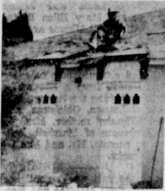
NEW STOOP — Part of the remodeling plans for Singleton Funeral home include a new entranceway. Here Noah Kinsler is shown at work on the new stoop.
