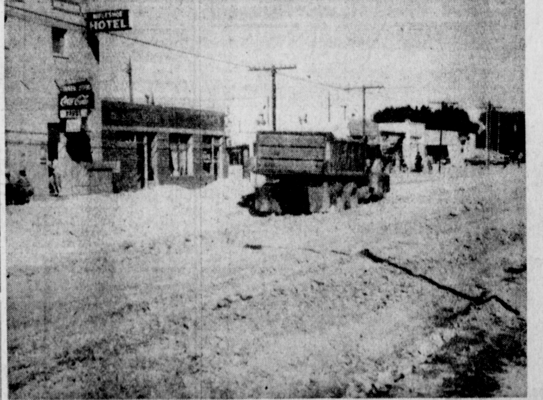
RE-PAVING the block west of Main Street sewer drainage system for the street, on Avenue B was begun last week, the final step in the installation of the storm (Journal photo and engraving)
