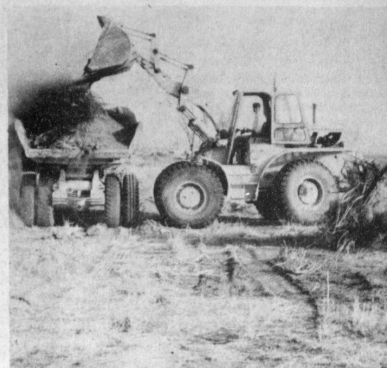
HAULED AWAY —The remaining debris from buildings, signs and other things are being loaded into dump trucks and hauled away. Graders are also at work along the route.
