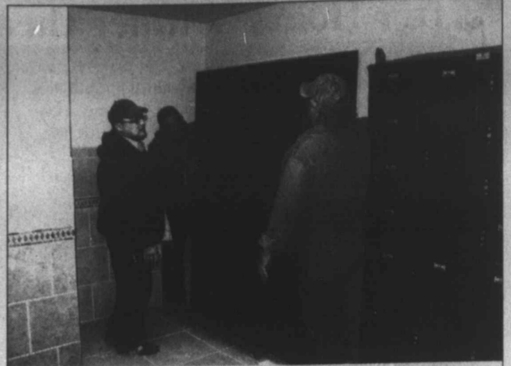
New lockers ... Lynn County Hospital District employee Felix Perez (left) and Wildcat Mfg. employees Libert Castillo and Todd Holland (right) install new lockers made at Wildcat for the new locker rooms at the newly remodeled LCHD Fitness Center and Family Wellness Clinic, which will open in mid-March.
