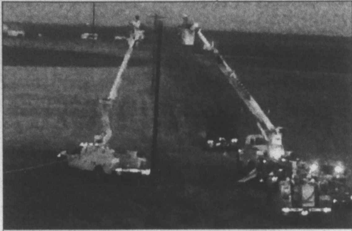
Working overtime ... Lyntegar employees worked throughout the weekend to repair electrical lines in many areas after thunderstorms caused power outages. This photo, taken June 5, was after a thunderstorm collapse with high winds near Pleasant Hill (6 miles west of Wellman) that took out poles and power lines and shut off power to 542 meters at Pleasant Hill and Jess Smith Substations (Seagraves). There were 20 linemen working diligently Saturday and Sunday to replace lines or backfeed from other substations to get the electricity back on as quickly as possible in the Lyntegar service area. The crews worked 350 hours between the 20 linemen, and there were 11 trucks out working. Lyntegar reported between 30-40 poles down from the storm.
