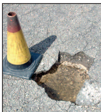
One of the holes in the coliseum's parking lot.
